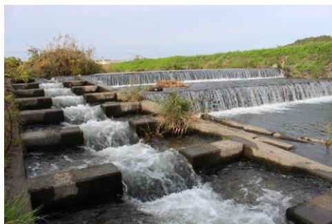
Fig. 2 Fish ladder (Juo River)
